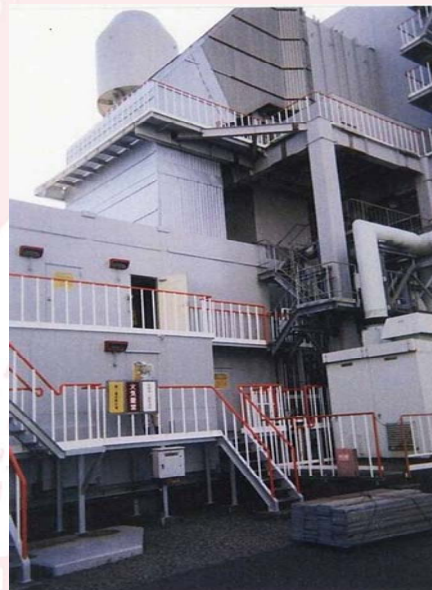
Air inlet duct
