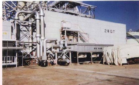
Exhaust Noise Control Wall
