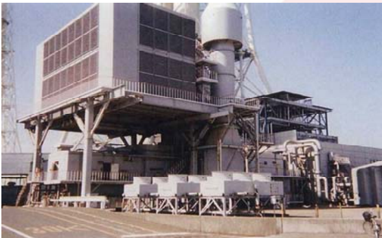
MW-701D GAS TURBINE POWER PLANT
